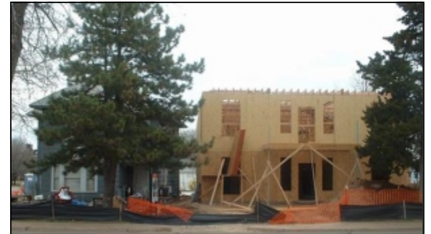
The new TKE House, under construction at 303 E. Ayers soon will be the home for 16 undergraduate Fraters who can start settling in this August. The house next door on left, where Tekes have made history for 25 years, is scheduled for demolition or sale and removal.
